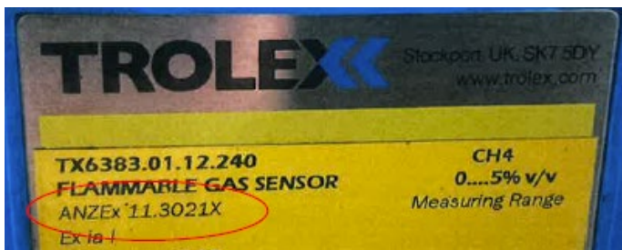
INCORRECT ANZEx LABEL
